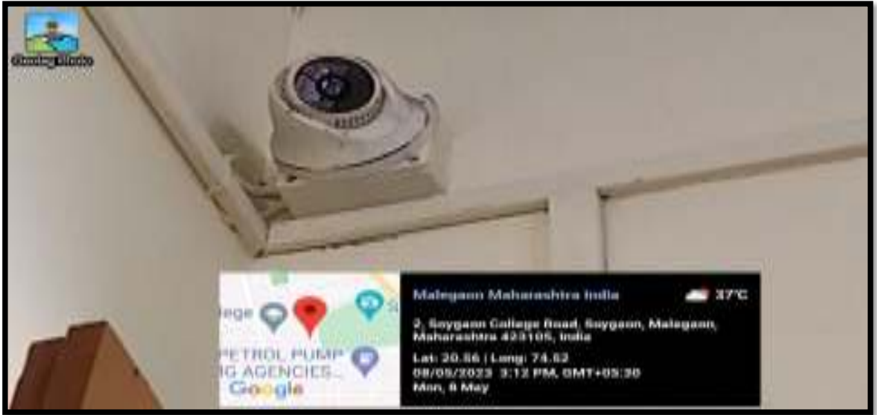
Exam Section CCTV Camera
